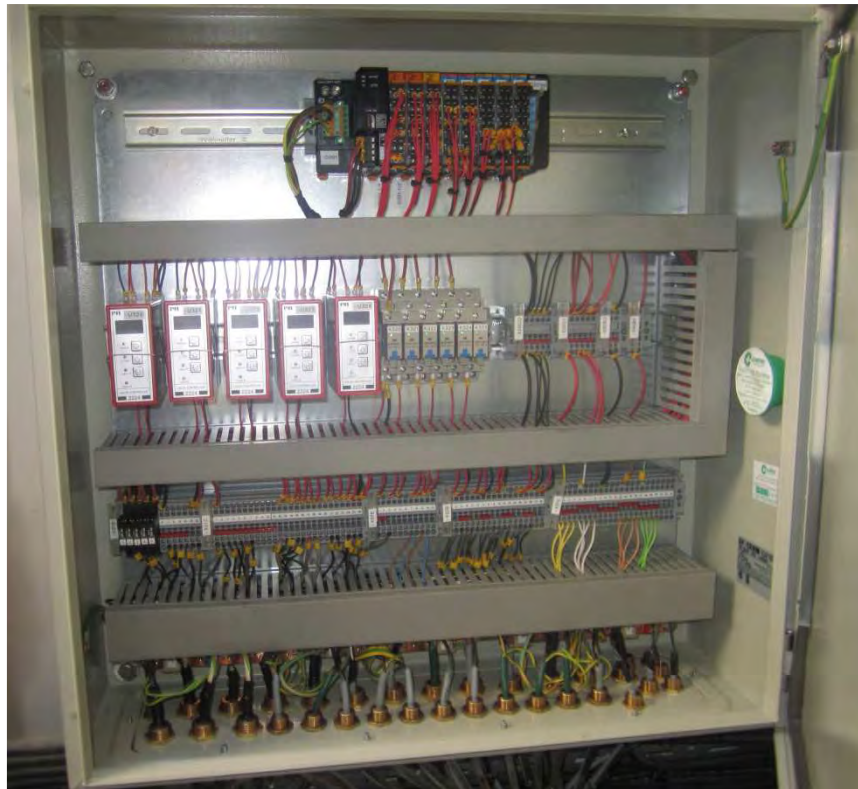
Figure 5-3 Control Cabinet –A140
